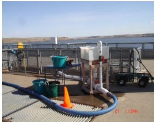
Figure 2: Planned fish release pipes design and method of attachment to traveling fish screen frame (top left photo) 30 inches off-center toward the north. Normandeau recommends that pipe design and installation (provided by Corp) follow that utilized previously in the 2007 study. The exit end of release pipes were curved (top right photo) and oriented in a downstream direction when installed. Normandeau will provide the same type of induction system and release hoses (bottom photo) used in 2007.
